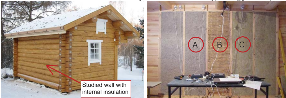
FIG 1. View of the test house from the back (left) and internally insulated wall (right).
