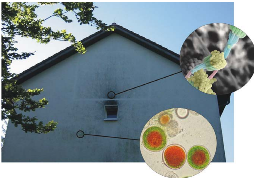
Figure 1. Growth of algae on a façade with external thermal insulation composite system (ETICS) and fungal growth above the window.
